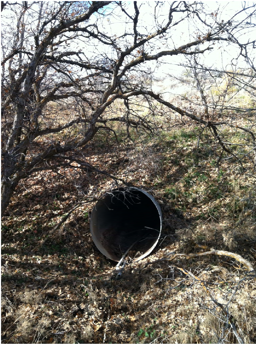
Photograph 5, taken on October 30, 2013, and looking west toward KUC showing the outlet of the existing 48-inch CMP draining the north fork of Copper Creek beneath U-111.
