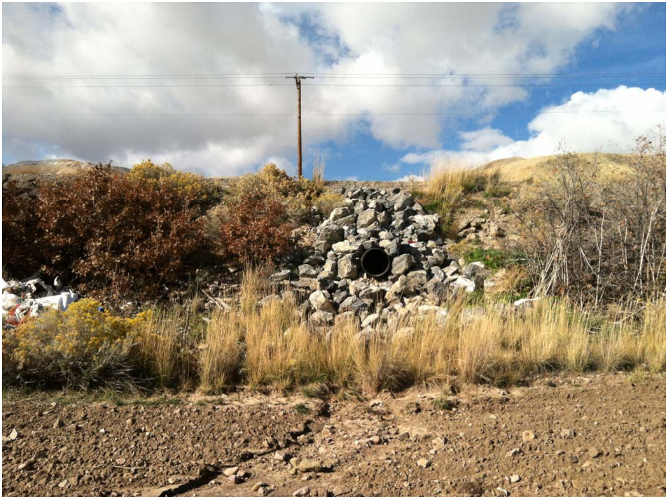
Photograph 6, taken on October 30, 2013, and looking west toward KUC and showing the HDPE pipe outlet draining Copper Creek proper beneath U-111. This pipe appears to be concrete on the upstream end.
