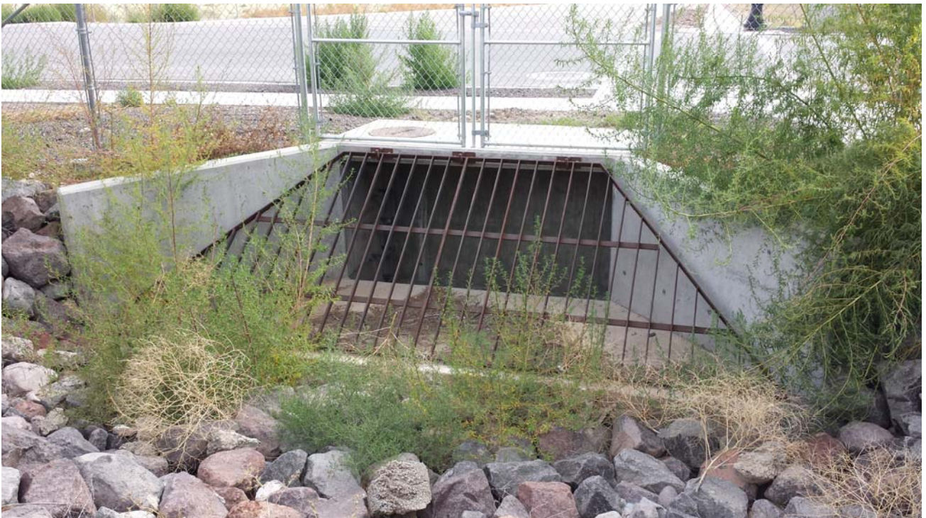
Photograph 2, taken October 2, 2013, looking east toward 6000 West. The drainage inlet structure designed as part of SWCCS project MC-1 to receive Copper Creek flows, which are then conveyed via pipe and channel to Midas Creek. Capacity of pipe as shown on the County construction drawings is 225 cfs.
